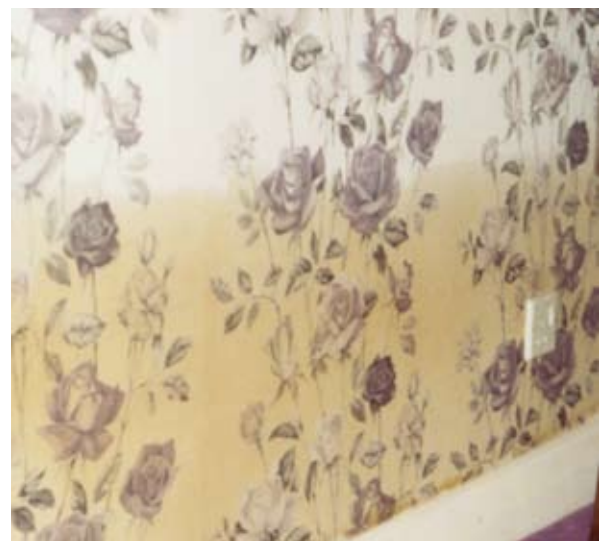
Figure 1: Staining to wallpaper on a wall affected by rising damp
