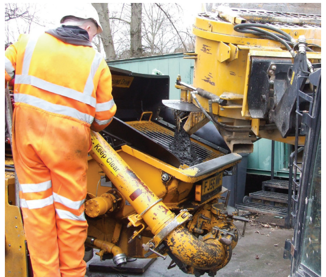
Figure 1: Alkali-activated binder concrete in industrial pumping trial to place piling concrete for aggressive ground conditions
