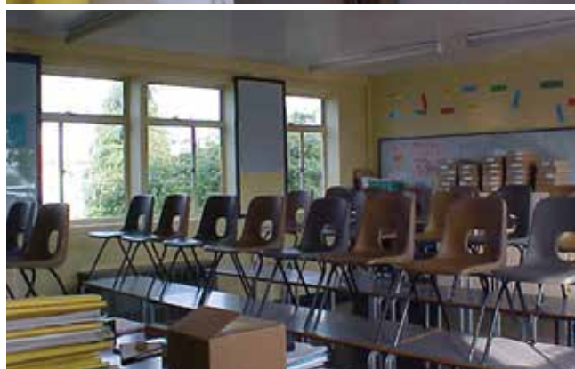
Figure 1: The improved condition of buildings enhances their suitability for teaching and learning
