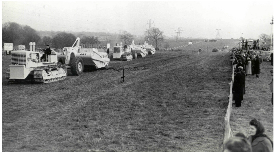
Figure 1.10 “Cutting the first sod”: removal of topsoil in preparation for embankment construction on the M1 south of Luton-Watford Gap Dunchurch Special Road Scheme (March 1958) (courtesy Owen Williams Ltd)
