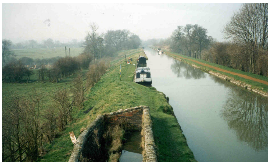
Figure 1.3 Canal embankment. Typically, water is retained by a lining. Although traditionally puddle clay was used for this purpose, replacement often utilises modern materials (courtesy British Waterways Technical Services)
