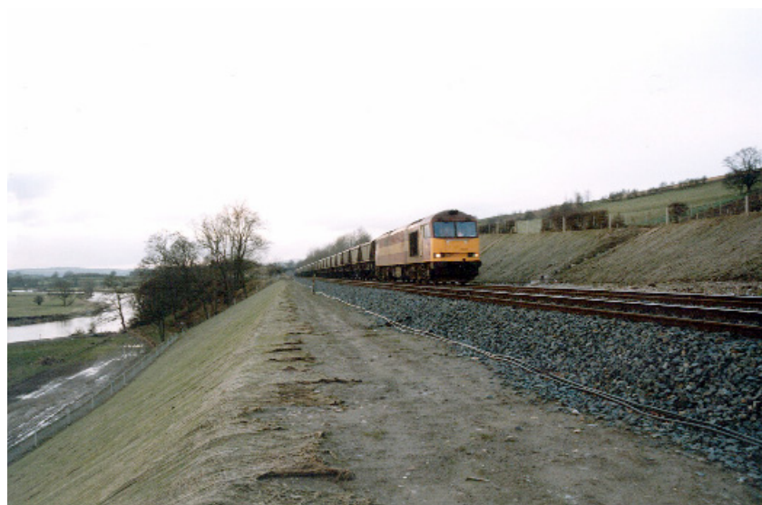
Figure 1.6 An example of infrastructure on sidelong ground, in this case a railway with tracks supported on a repaired slope (courtesy Network Rail)
