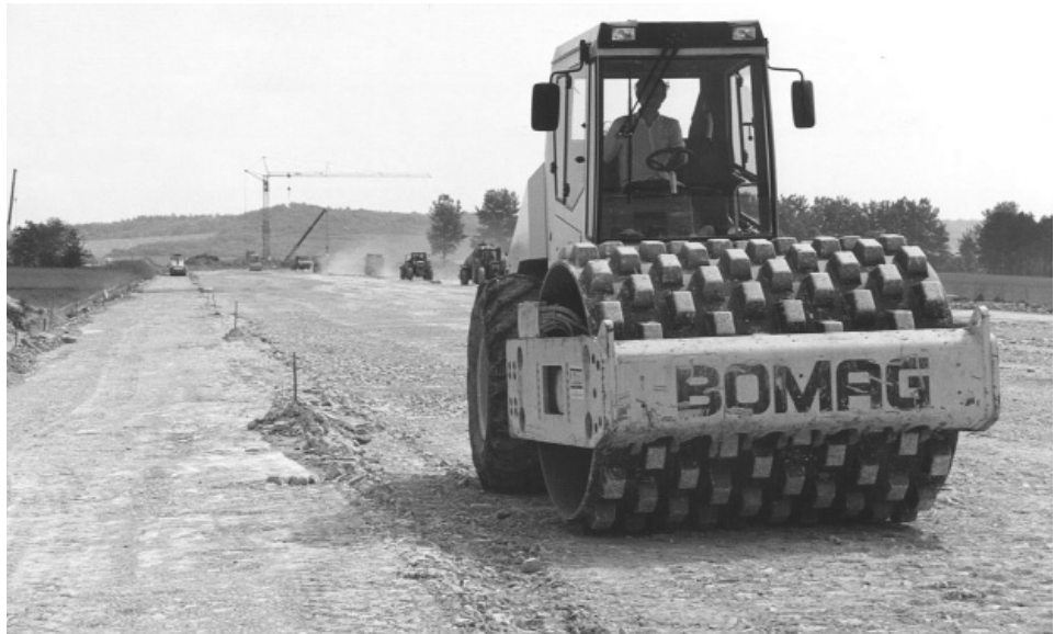
Figure 1.11 Use of modern and efficient compaction plant on a recent highway embankment (courtesy Bomag (GB) Ltd)
