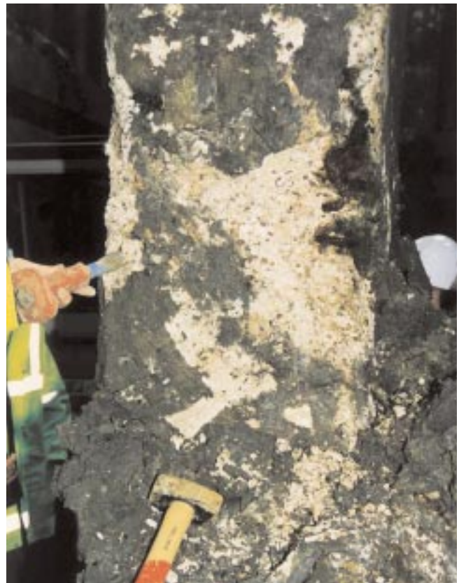
Figure A1 Extreme example of sulfate attack in a 30-year-old highway bridge sub-structure exposed to wet, pyritic clay fill
