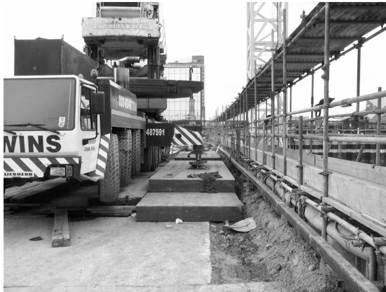
Figure 1.9 Tower crane erection requires careful planning to ensure that access is available
