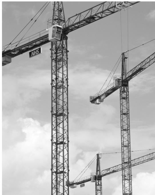
Figure 1.2 Proximity hazards (Photo courtesy HTC Plant Ltd)
