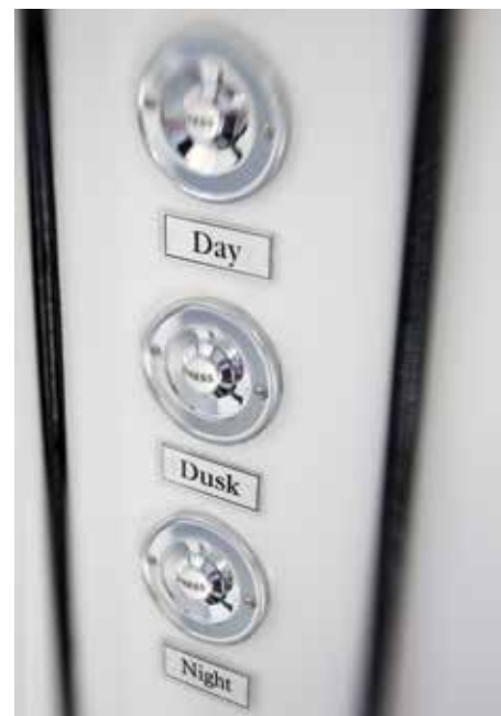
Flexible controls, used in a retail setting, allow shoppers to change lighting settings in the fitting rooms, between simulated 'day', 'dusk' and 'night' (© Boux Avenue)
