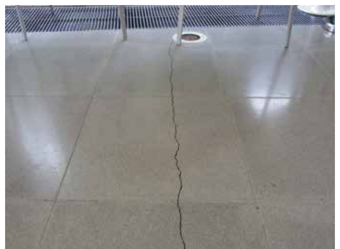
Figure 2: Crack spanning multiple tiles
