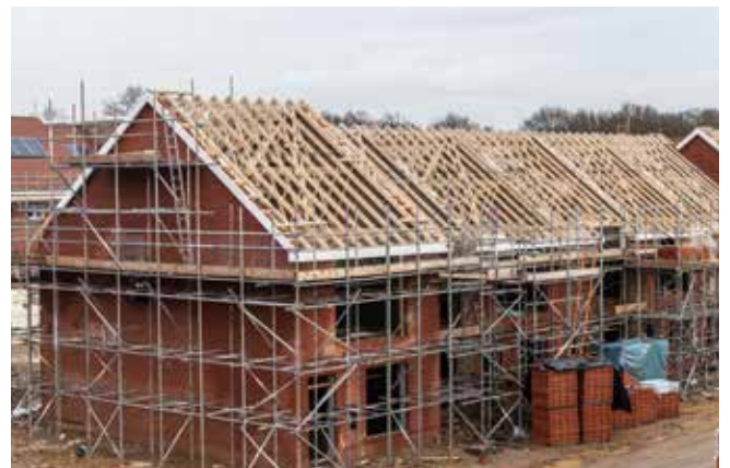
Figure 1: Sound insulation must be considered throughout the building process for new homes
