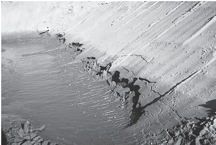
a) Slumping of side slopes caused by seepage into an excavation in fine sands
