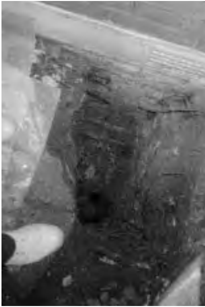
Figure 2.26 A narrow diameter hole has been excavated in a confined space alongside a one brick solid external wall to establish the depth and width of what turned out to be brick footings. Both depth and width had to be established by probing with a long crowbar. The footings were on shrinkable clay, and were unusually deep for an Edwardian house. Tree roots are visible in the sides of the excavation
