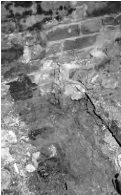
Figure 2.27 A variety of contaminants has obviously been in contact with this 100 year old clay brickwork below DPC level, but only minor damage has resulted. There is also evidence of previous alterations and some repointing
