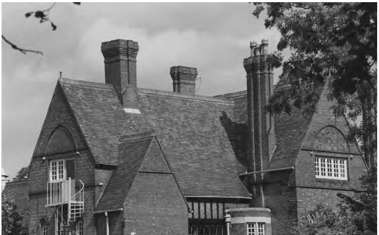
Figure 3.1 This steeply pitched plain tiled roof was built in 1880 but re-covered after bomb damage in the 1939–45 war
