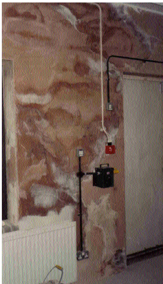
Figure 5.3 Severe wetting from driving rain on an exposed wall
