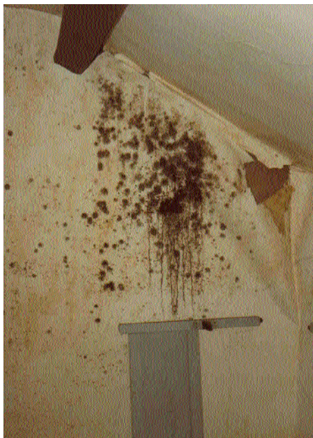
Figure 5.2 Although much of this results from condensation, there is also some rain penetration
