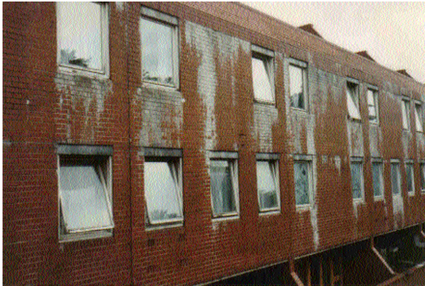
Figure 5.1 A disfiguring deposit of carbonate from rain penetrating the sloping brickwork parapet
