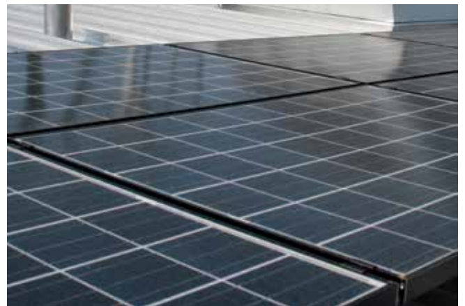
A photovoltaic system on a flat roof
