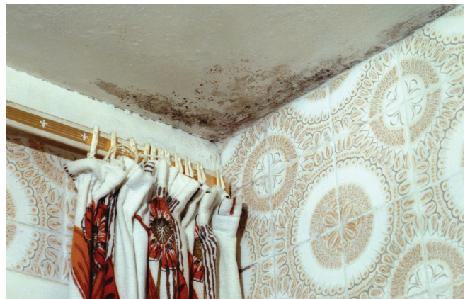
Figure 1: Typical example of mould caused by condensation
